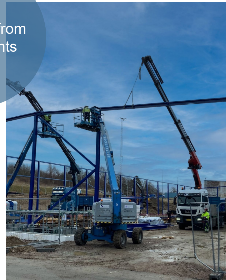
New press hall for Lindab Ventilation in Grevie (SE), is being erected.
